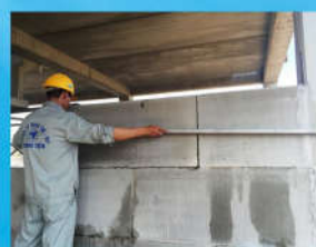
Use a long bar to check the flatness of the wall during erection
